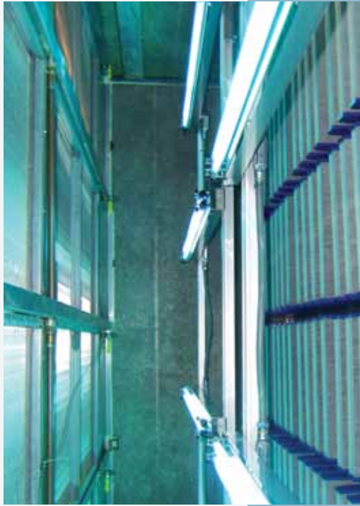
American Ultraviolet UVC lamps inside an air handling unit
