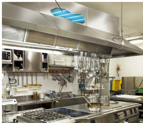
KE Series UV lights installed in kitchen exhaust plenum
