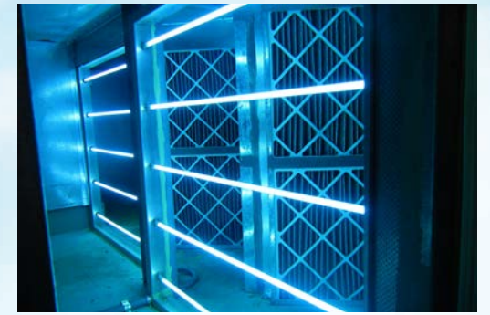
High Intensity UVC Rack Inside Air Handling Unit
