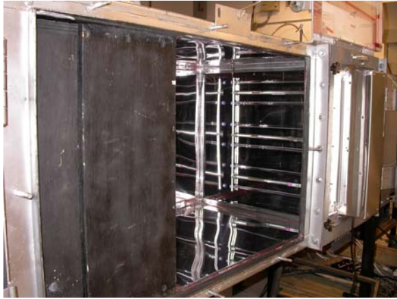
Figure 2-1. Ballast box installed on the outside of the test rig (on right). The device is also visible.
